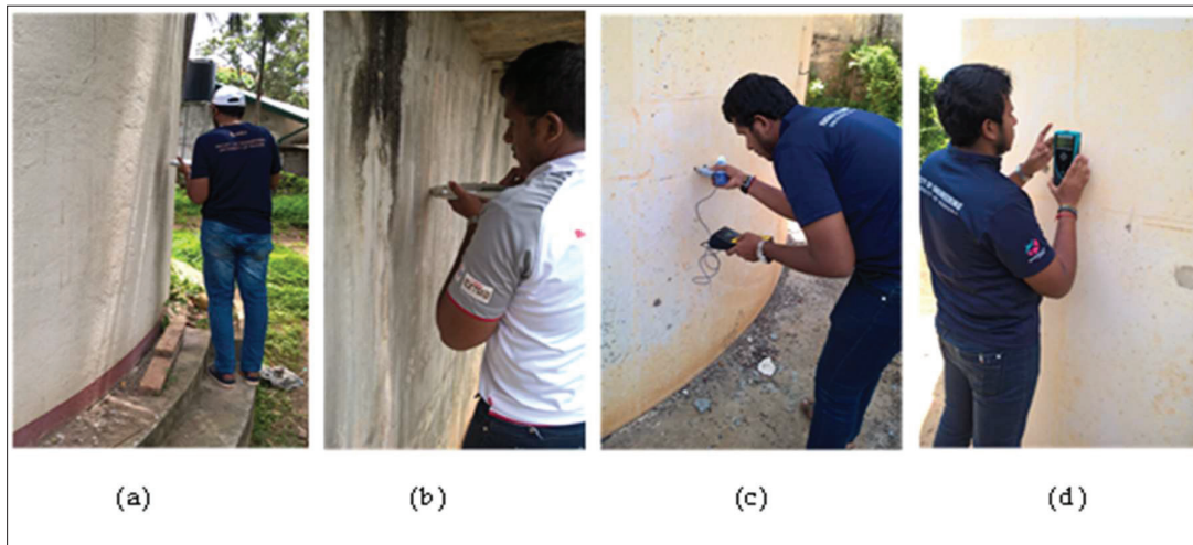
Figure 3: Data collection by NDT: (a) record data from visual inspection; (b) rebound hammer test; (c) concrete resistivity test; and (d) cover meter survey
