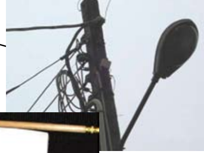
Device installed on street lamp
